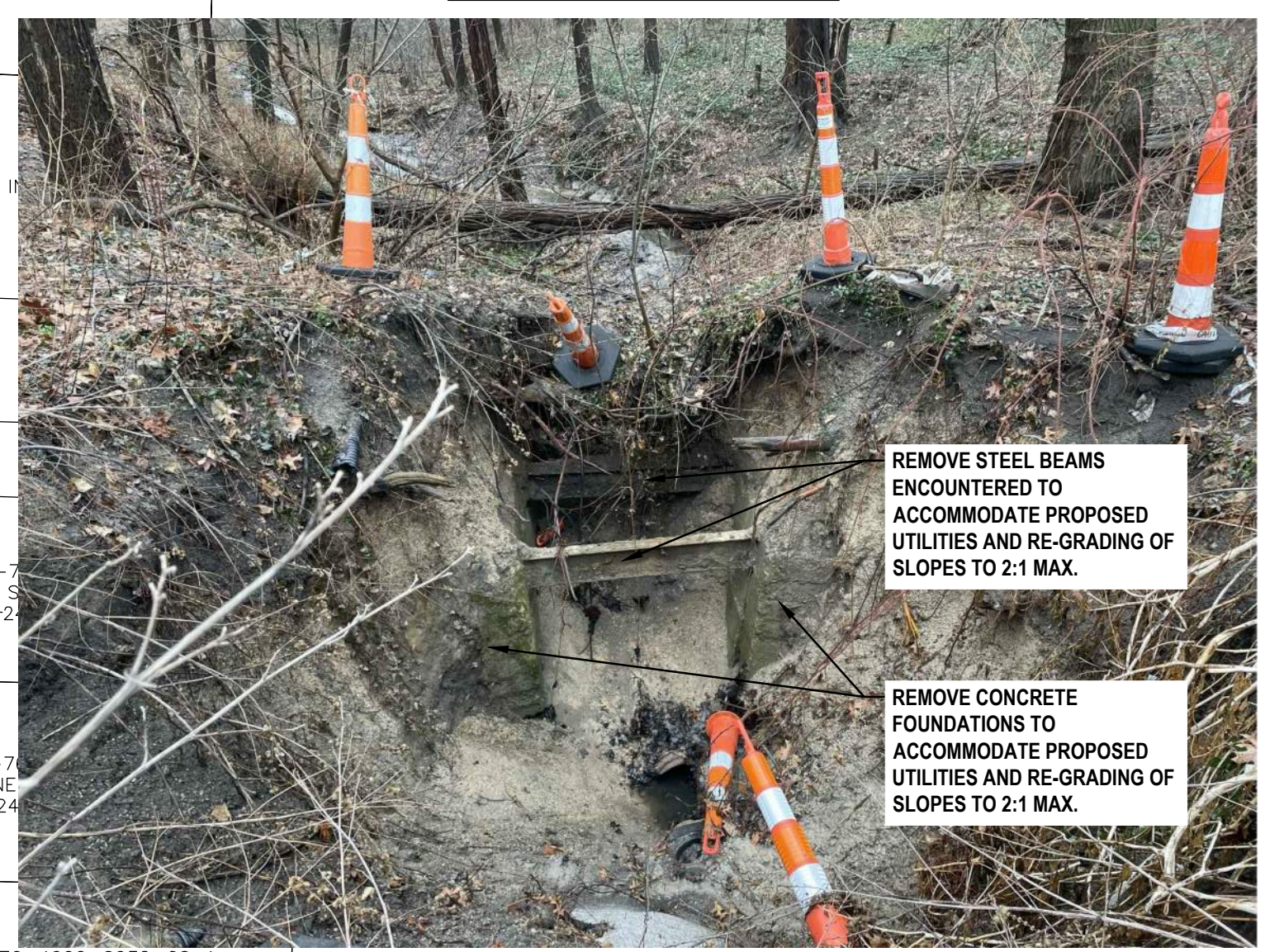
PHOTO OF EXISTING CONCRETE FOUNDATIONS AND BEAMS TO BE REMOVED (VIEW LOOKING SOUTH)
